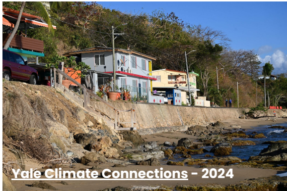
Accelerated coastal erosion post Hurricane Maria
